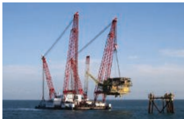
Overdick's operational concept saw the Welland platform removed in just two lifts – one for the topside and one for the jacket and the piles.
